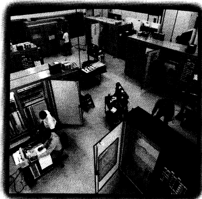
An overview of the room at Universal where technicians build and test the company's automation control panels.
