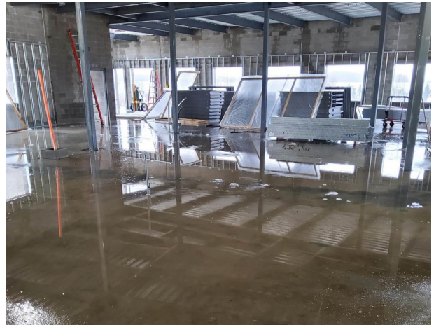
Photo 1. Flooding on a job site can stall productivity.
