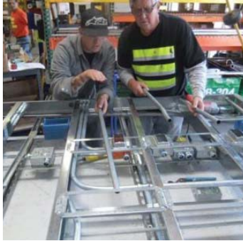
Photo 2. Had the electrical contractor not seen an opportunity to prefabricate the entire headwall as a preassembled section, then all of the work would have been completed on the job site as originally scheduled. Recognizing this opportunity saved thousands of hours.
