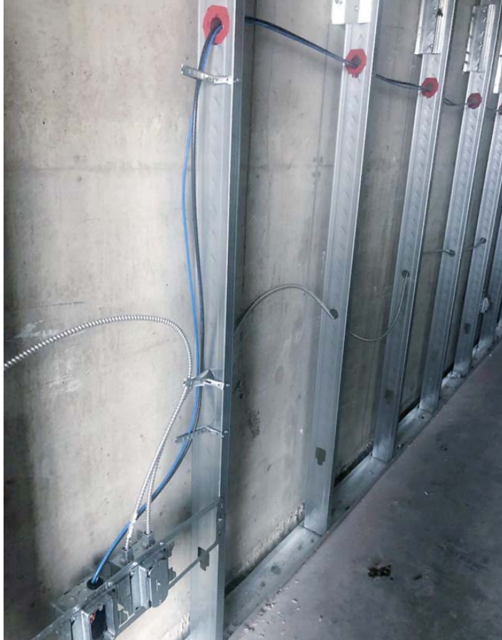
Photo 3. In this example, there are both low-voltage and electrical branch wiring present. Both scopes were done by the same company and installers but conducted in two passes. This work could have been combined into a single pass, using far less material-handling effort.
