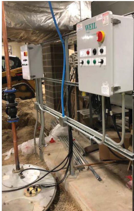
Photo 1. This is an example of overbuilding by running control wiring for HVAC equipment outside of the electrical scope, which was done as a favor to the mechanical contractor who was responsible for this scope of work.
